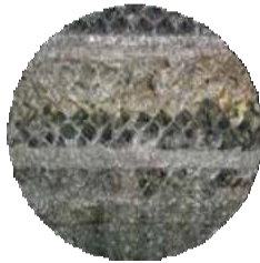
Check the components inside the oil separator and clean them if necessary
